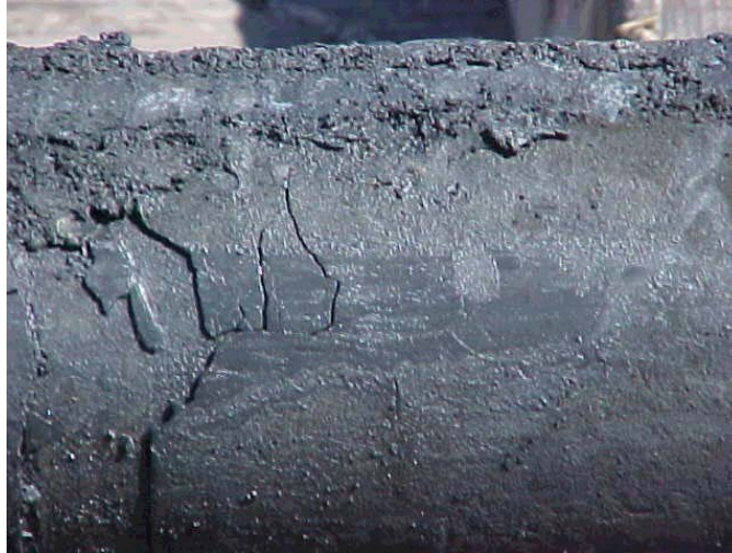
Figure 5 - Another View of Scale and Produced Solids Bonded to the ESP Motor
