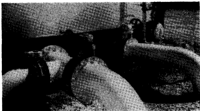
FIG. 9—WATERFLOODING - ISOLATION VALVES FOR FILTERS
