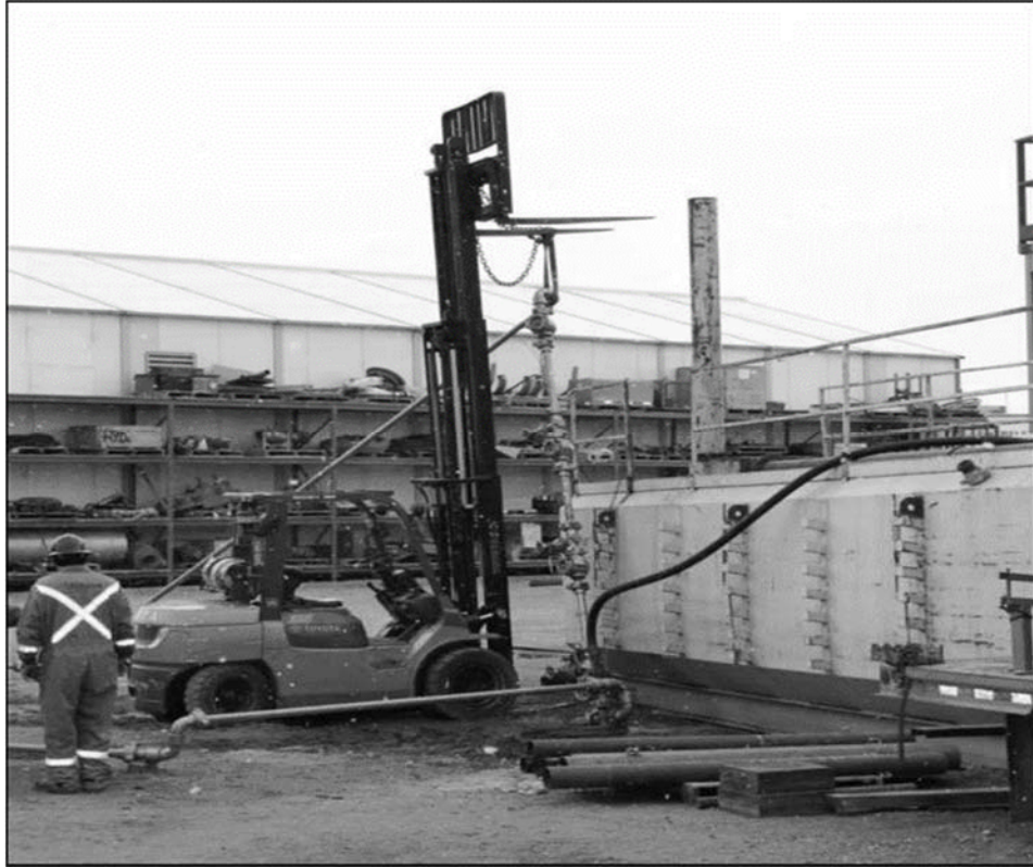
Figure 11 - Vertical stand of pipe and sample valves for high-pressure suspension test.
