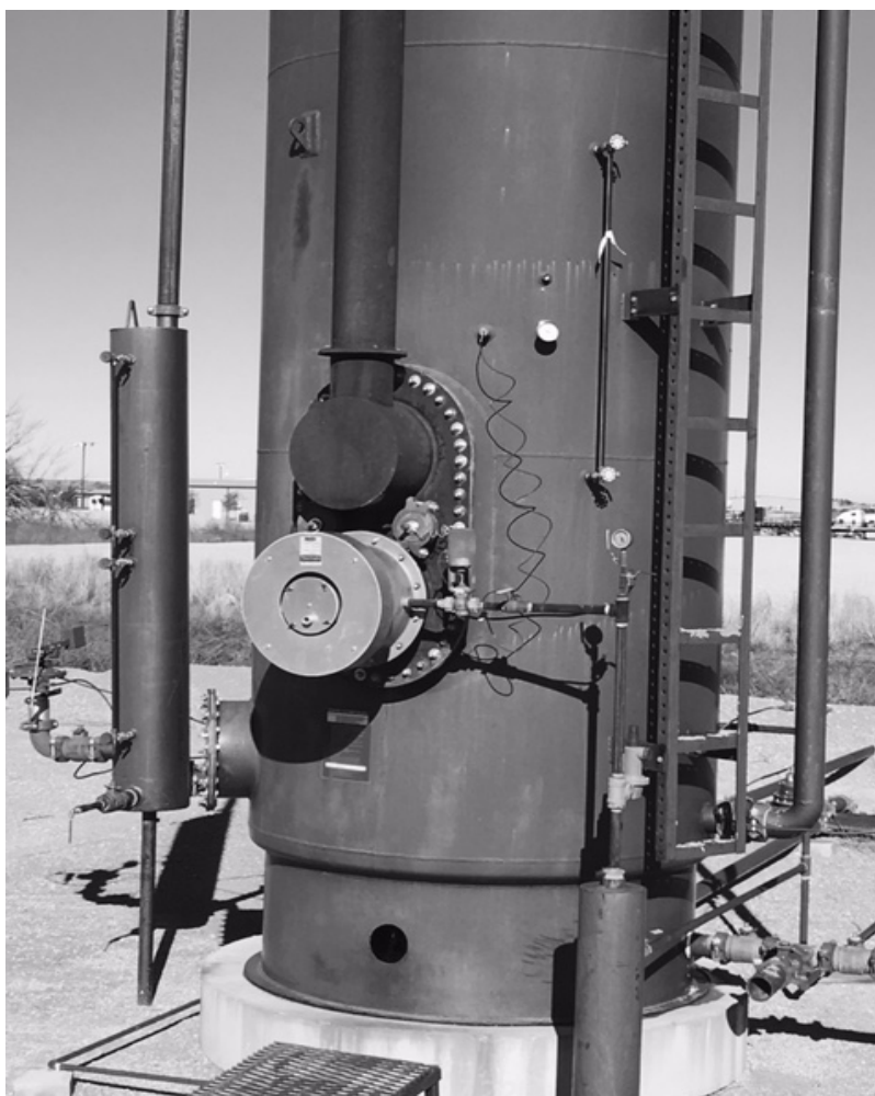
Figure 1 – Sight glass marker used to determine fluid retention in heater-treater
