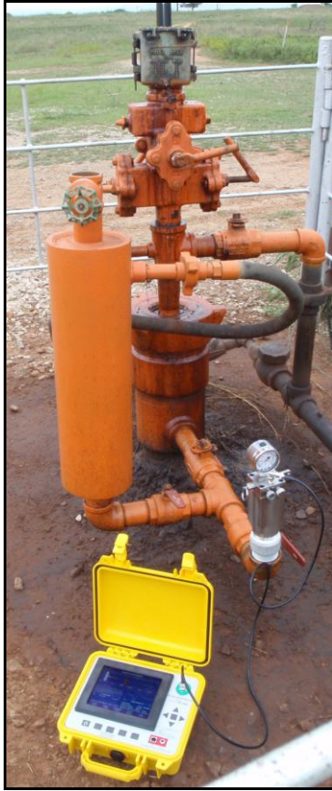
Figure 2 – The Echometer Model H Installed at the Wellhead with an Intrinsically Safe Acoustic Pulse Generator
