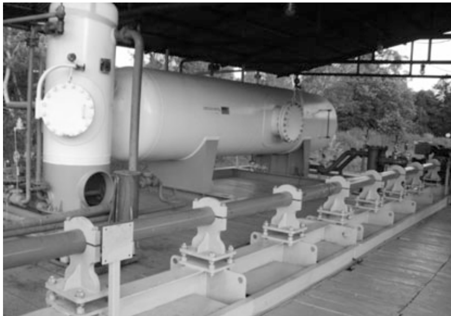
Figure 8.0 The first HPS installed in 2008 and operated until 2021 with only two thrust chamber mechanical seal failures.
