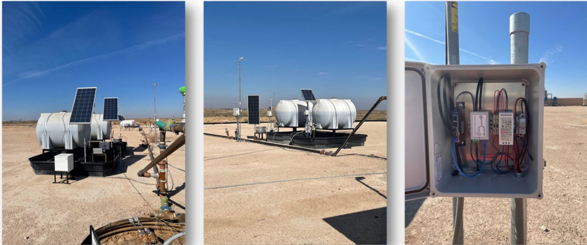
Figure 1 – Images of the chemical tanks, solar panels, chemical pumps, and controllers used at one of the producing wells in the pilot project.
