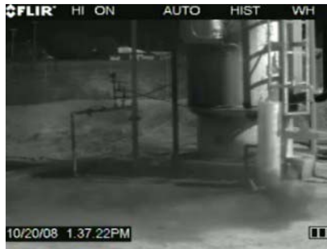
Picture 1 -Leak on a scrub pot that supplies gas to water and oil dumps.
