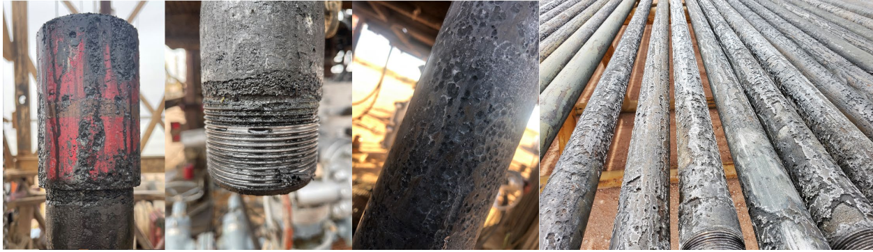
Figure 1 – Corrosion morphology in annular flow wells from Bone Spring and Wolfcamp formations in the Delaware Basin
