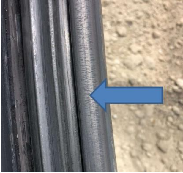
Figure 10: Well No. 2 - Stress Cracking
