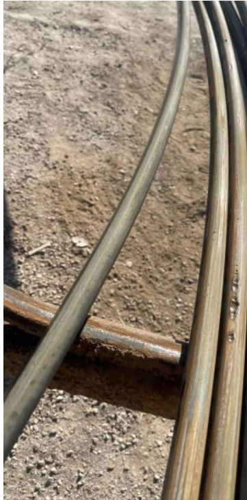
Figure 13: Well No.3 - Moderate to Severe Pitting
