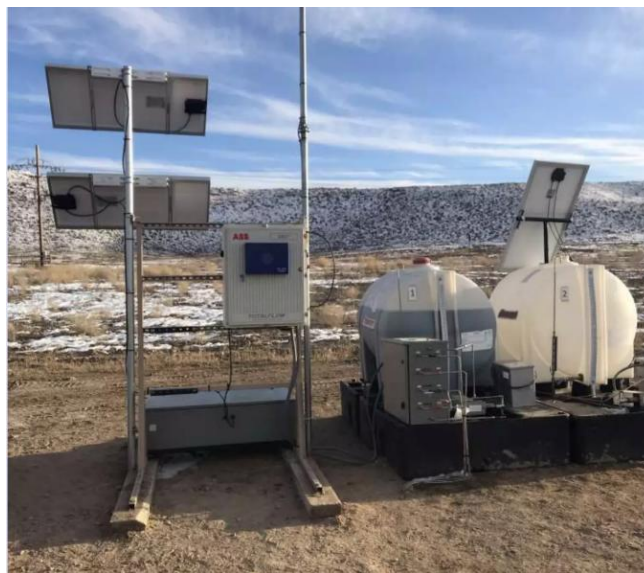
Figure 15: ABB TotalFlow system with solenoid header and controller for well pad.
