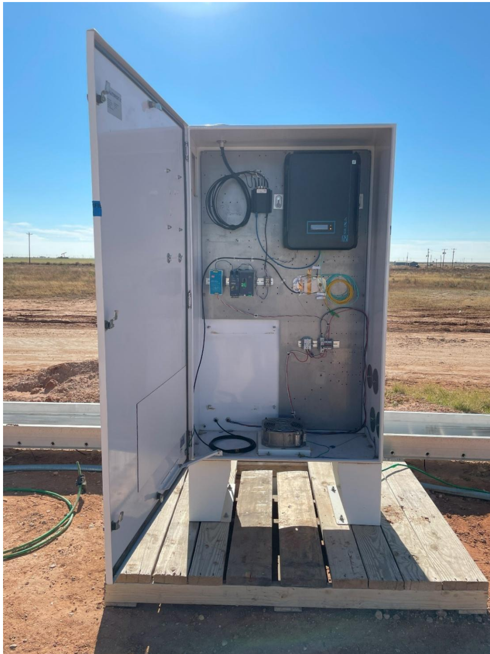
Figure 6. DTS Interrogator Enclosure. Source: SLB
