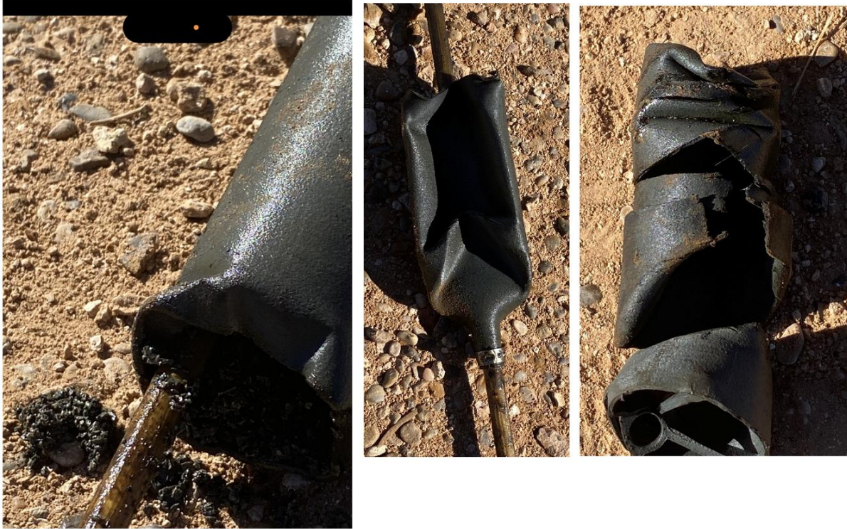
FIGURE 42 – MUDSHARK FAILURE DUE TO PUMP UNSEATING CASE STUDY
