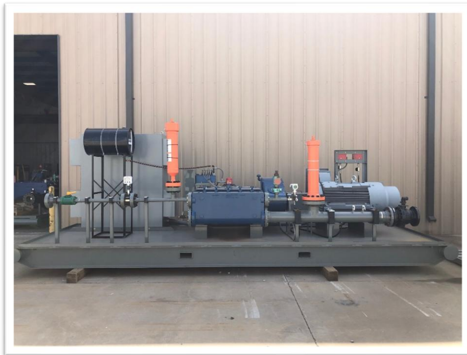
Figure 3: Power fluid unit or pump skid
