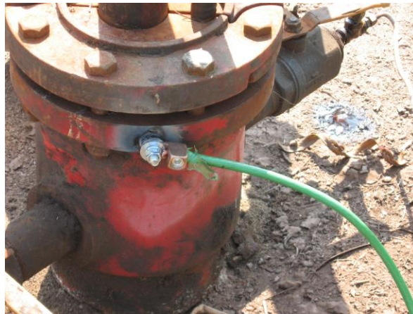
Figure 6a – Welded Bolt Head and Ground Lug
