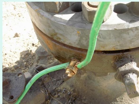
Figure 6b – Service Post Ground
