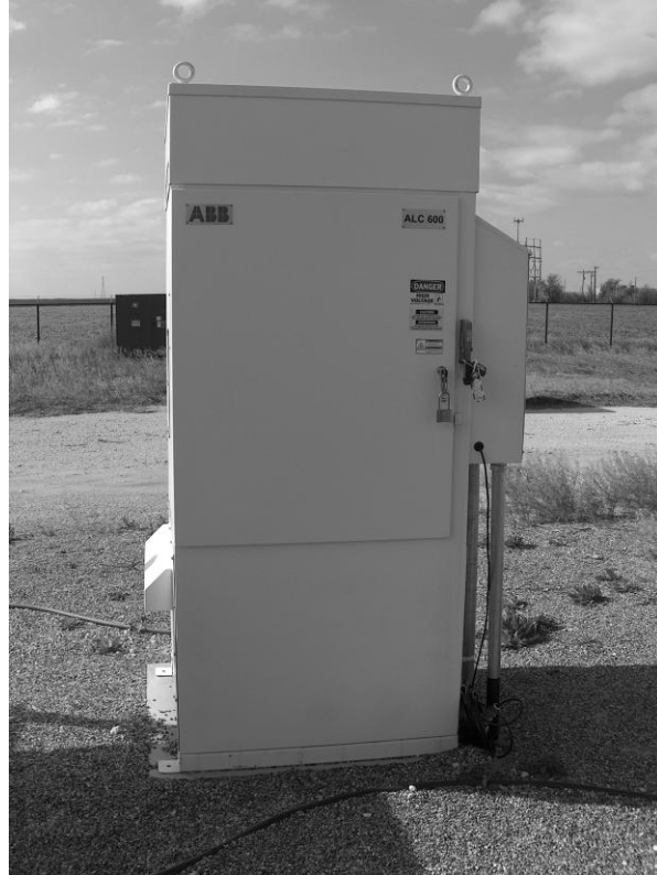
Figure 6 – ABB Variable Speed Drive
