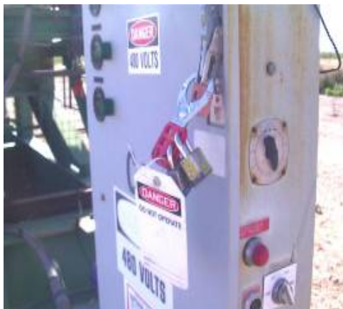
Lock and Tag Properly Placed on Disconnect
