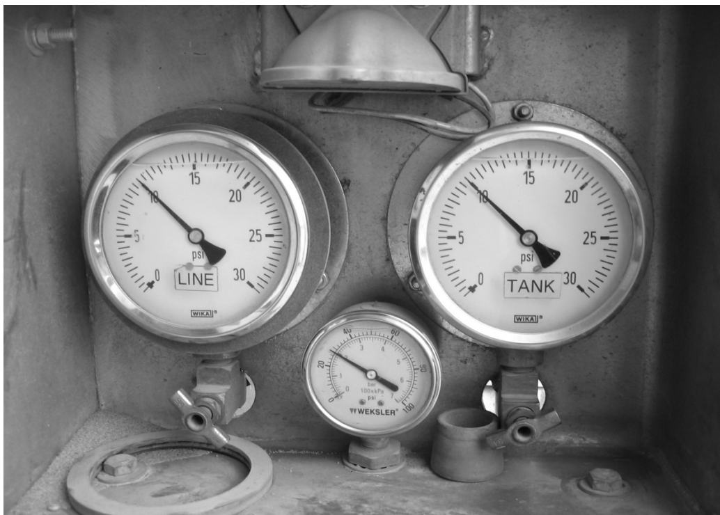
Figure 4 – Trailer Gauges for pneumatic pressure
